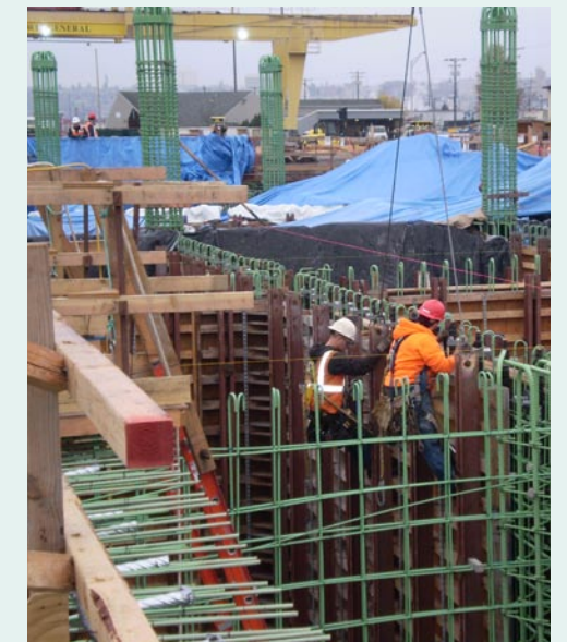
Carpenters set wall forms for pontoon ZD prior to a concrete pour, Nov. 28, 2007.
