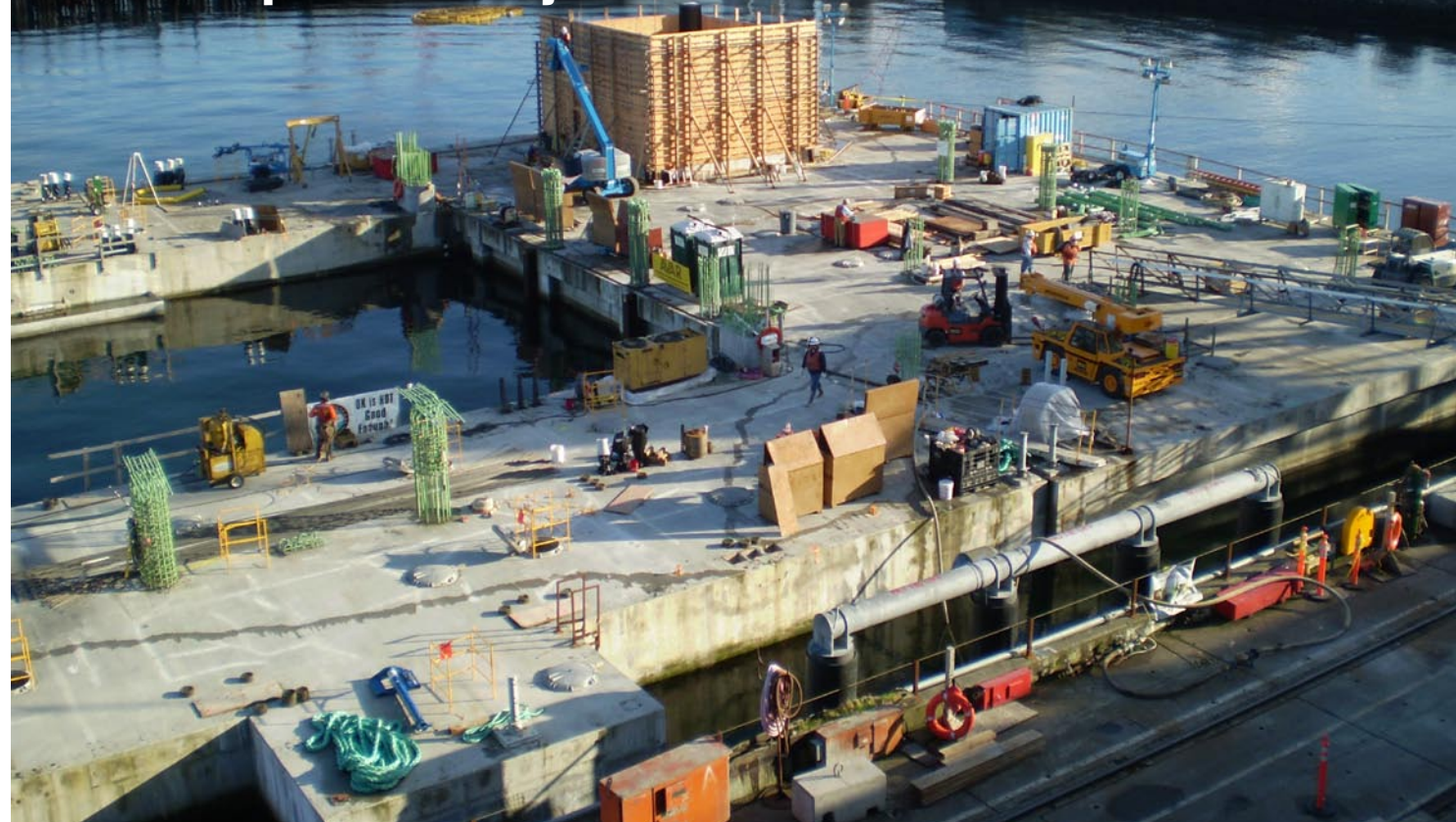
The electrical building forms are in place on the new east-half Hood Canal Bridge "U" shaped draw span, Dec, 31, 2007.
