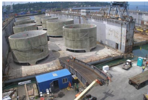
The last ten Hood Canal Bridge anchors are ready to be floated to the Hood Canal Bridge site, June 19, 2007.
