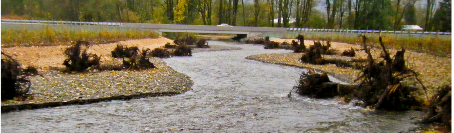
A barrier culvert was replaced in 2011 on SR 20 Red Cabin Creek with a 66-foot bridge.
