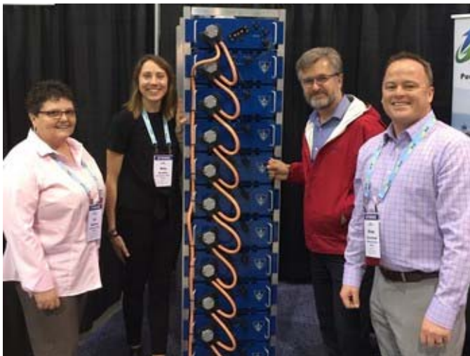
Checking out a bank of batteries such as those that could someday be used to power our ferries.
