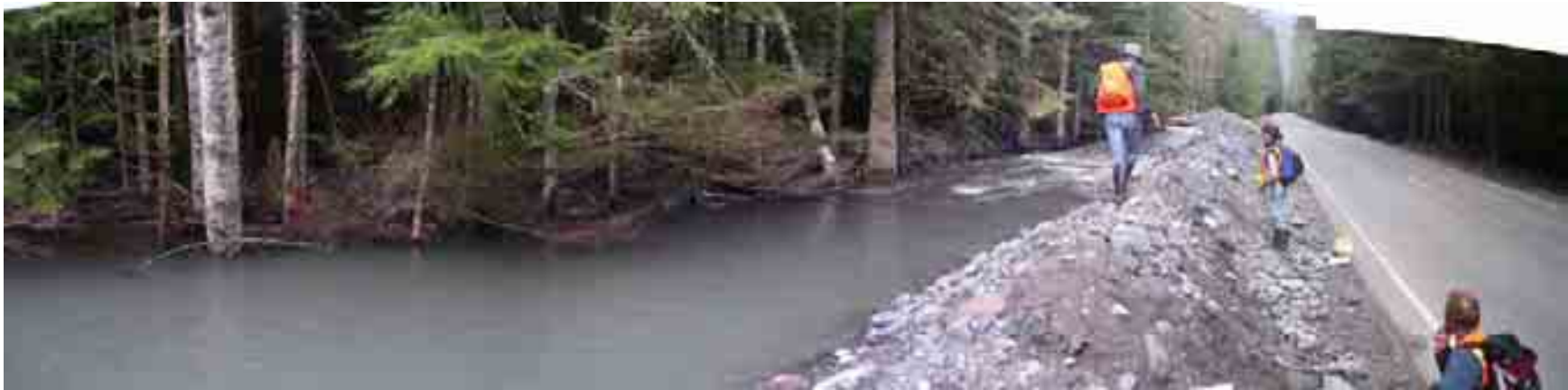
Upstream end of Site 4, MP 58.4. Location where river flow across floodplain currently encounters SR 410. Looking downstream (North) where emergency gravel dike separates side channel flow from highway. Water surface is approximately 1 foot above highway surface during low flow conditions. Note submerged trees to the left. April 27, 2005.
