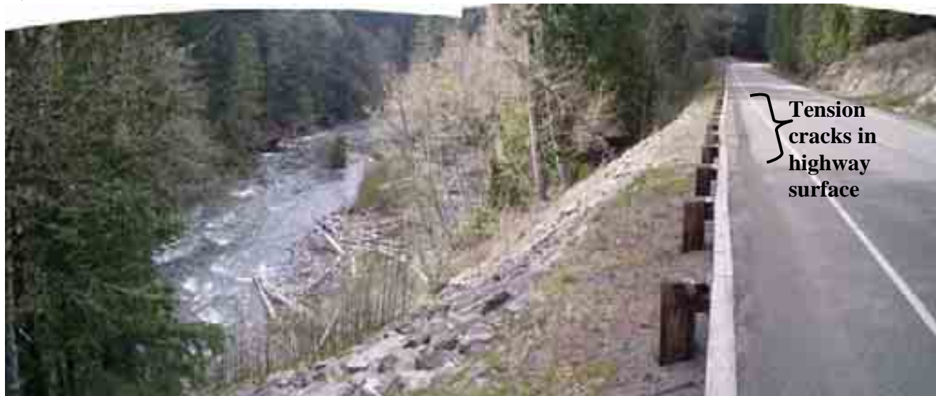
Site 3, MP 55 looking downstream of failing slope. April 25, 2005.
