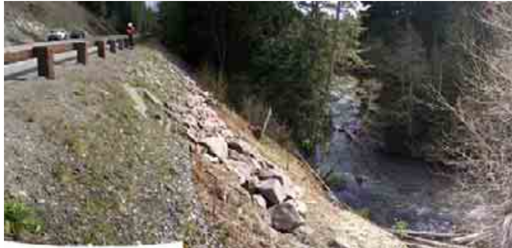
Site 3, MP 55 looking upstream of failing slope. Highway is situated approximately 70 ft above river. River is actively eroding toe of slope. April 25, 2005.
