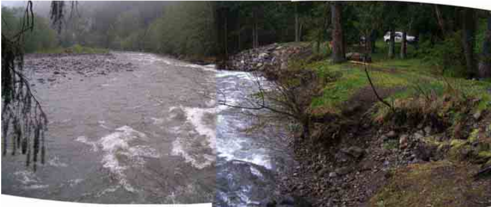
Site 1, Milepost 38 looking downstream at eroding right bank upstream of rock revetment. April 25, 2005.
