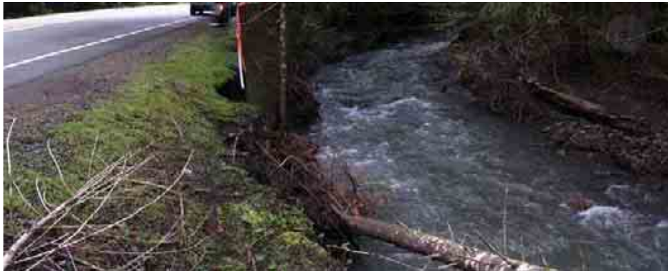
Site 4, MP 58. Looking upstream at side channel along SR 410 where on-going erosion threatens highway embankment. April 27, 2005.
