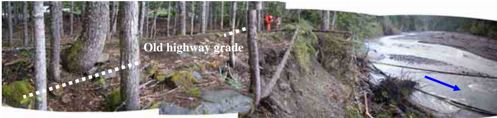
Site 7, MP 59.25. Looking upstream at eroding high bank along maintenance yard. April 27, 2005.
