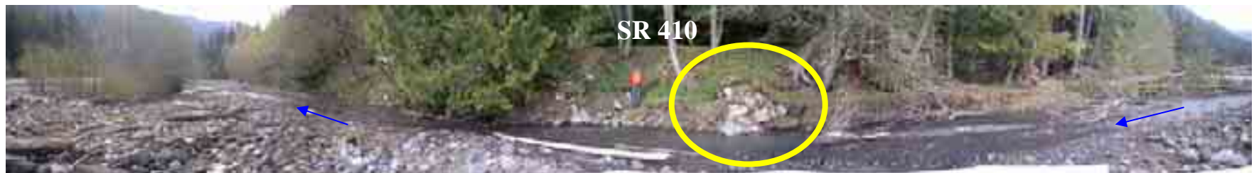
Site 6, MP 59. SR 410 highway embankment along mainstem of White River. Flow is from right to left. Note recent bank failure at center of photo. Recent tree recruitment to river at right may help to deflect flows away from road grade, but a series of ELJ structures is recommended to extend armored riparian forest buffer out from highway approximately 30 feet. April 27, 2005.
