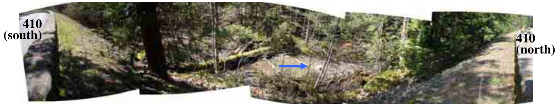
Site 2, MP 51.6. Side channel running along SR 410 embankment downstream of Skookum Falls Overlook. Engineered logjams and LWD armoring is recommended along toe of slope to keep erosive flows away from highway embankment. April 25, 2005.
