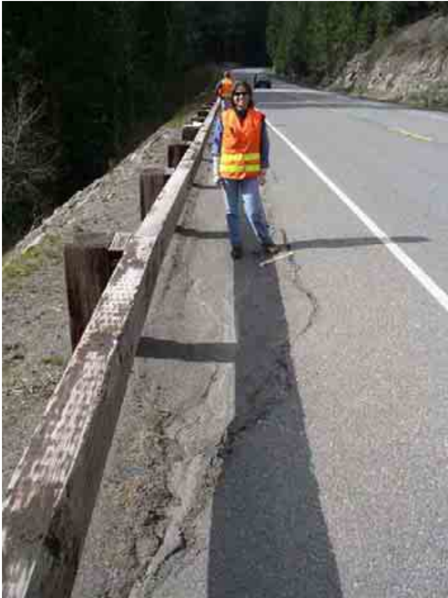
Site 3, MP 55 looking downstream at slope displacement and tension cracks in highway surface. April 25, 2005.
