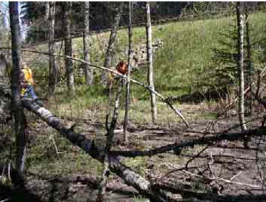
Site 2, Milepost 51.6. Looking downstream from side channel inlet at SR 410 embankment. April 25, 2005.
