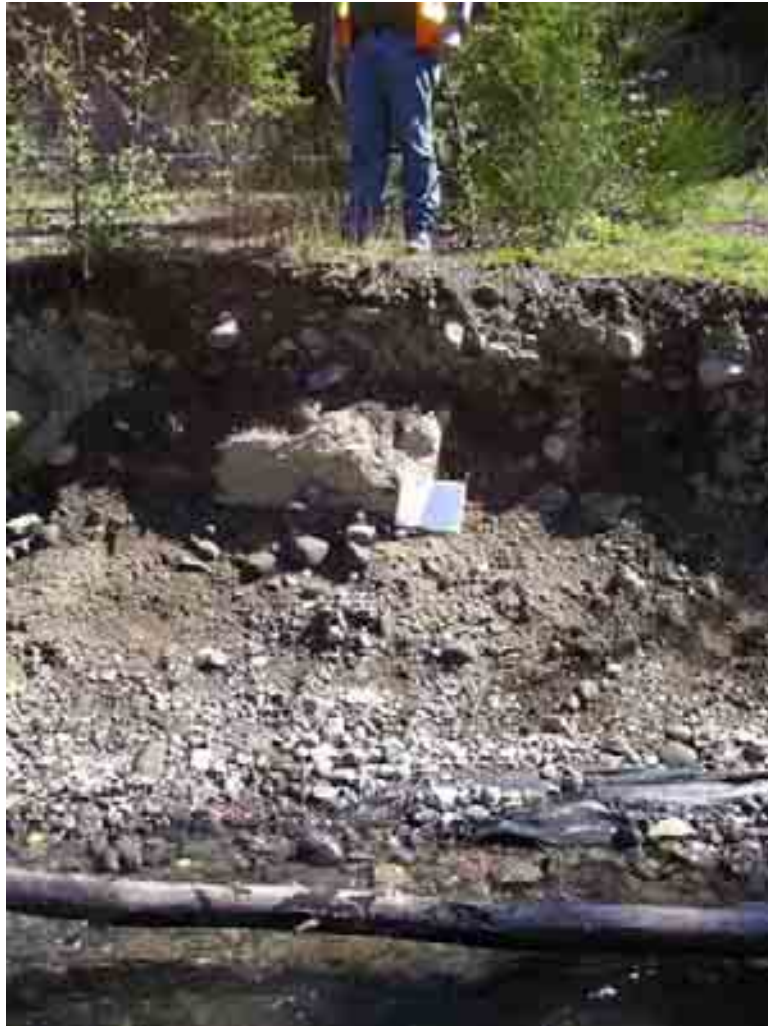
Site 2, Milepost 51.6, Skookum Falls Overlook eroding right bank. Note exposed geotextile at toe of bank installed in previous bank protection measures. April 25, 2005.
