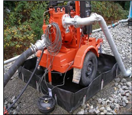
Secondary containment for equipment
