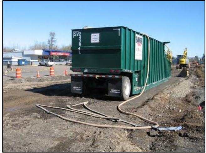
Contaminated ground or surface water collection and treatment in Baker tank.
