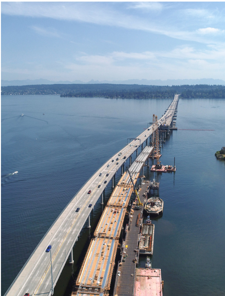
The new eastbound connection bridge takes shape on SR 520 cross Union Bay and Lake Washington in King County.
