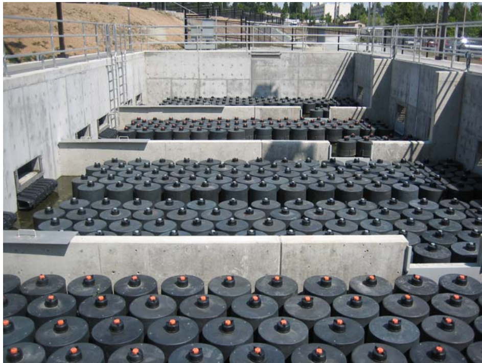
Underground media filter (Stormfilter) at SeaTac.
