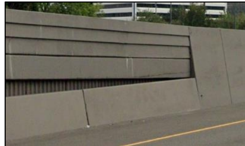
Photo B: Need for Mitigation - Single Slope Barrier Connecting to Tall Wall
