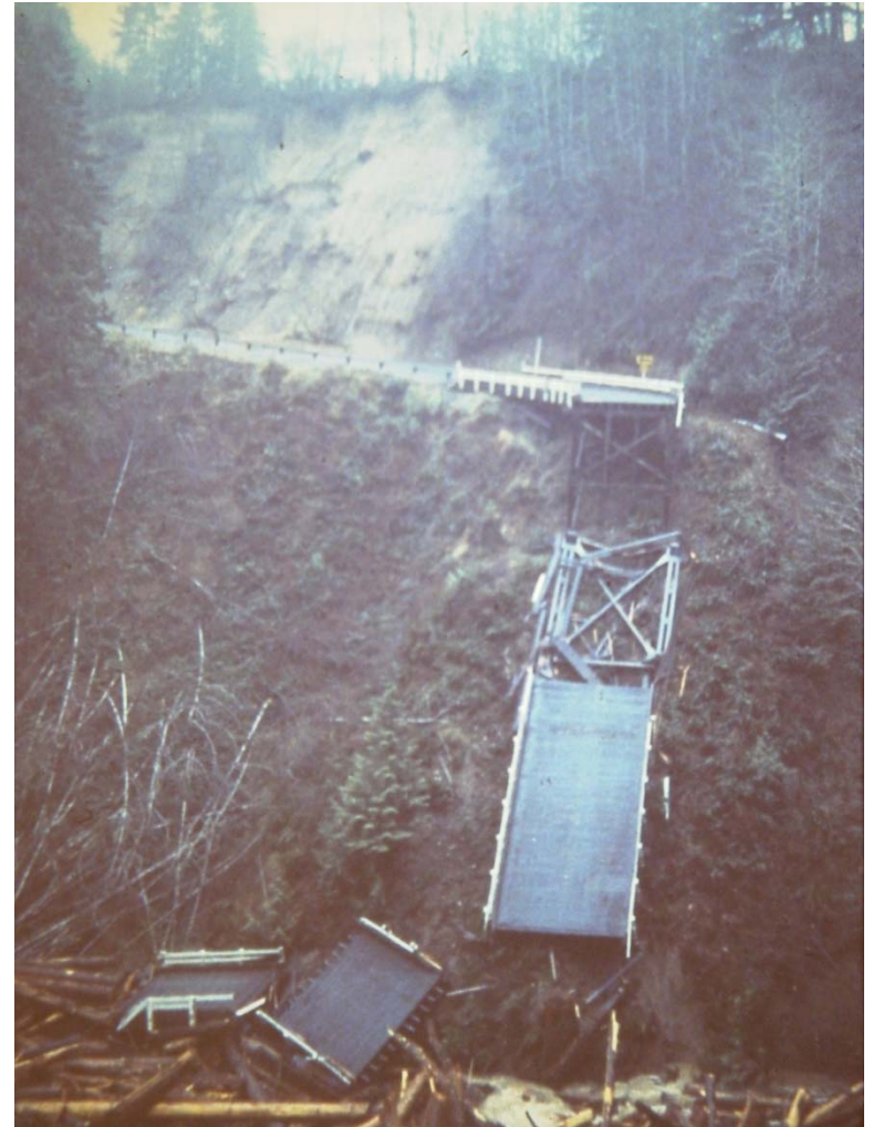
Location: SR 508 Bear Creek Cause: Flood/Debris bent center and 2 trusses
