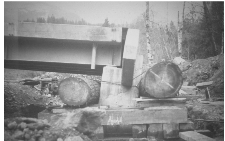
Location: SR 542 Gallup Creek Cause: Flood washed out abutment, dropped 4'6"; 1962
