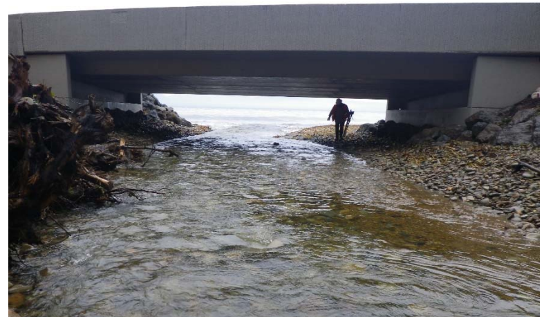
SR 112 Jansen Creek, built 2016
