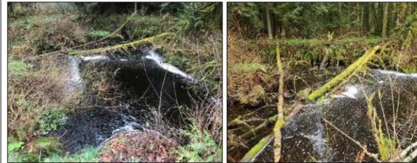
Figure 10 Scour pool above culvert outlet (left), scour pool from left bank (right)
