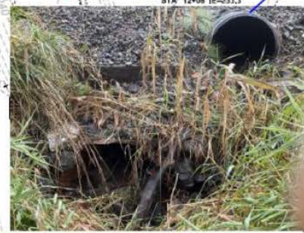
Private roadway culverts. 36-inch rusted corrugated metal pipe and 24-inch overflow pipe
