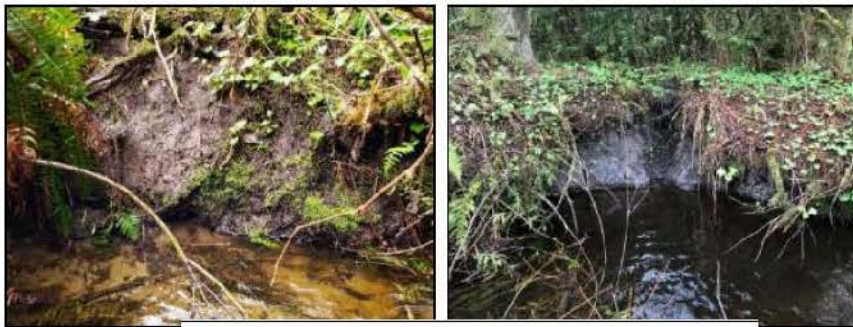
Figure 5 Erosion on right bank at 180 degree turn (left), groundwater seep (right)
