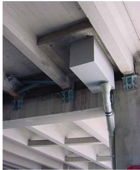
Figure RT.18.4. StormFilter™ catch basin in a bridge deck from under the bridge. (Courtesy Stormwater Management, Inc.)
