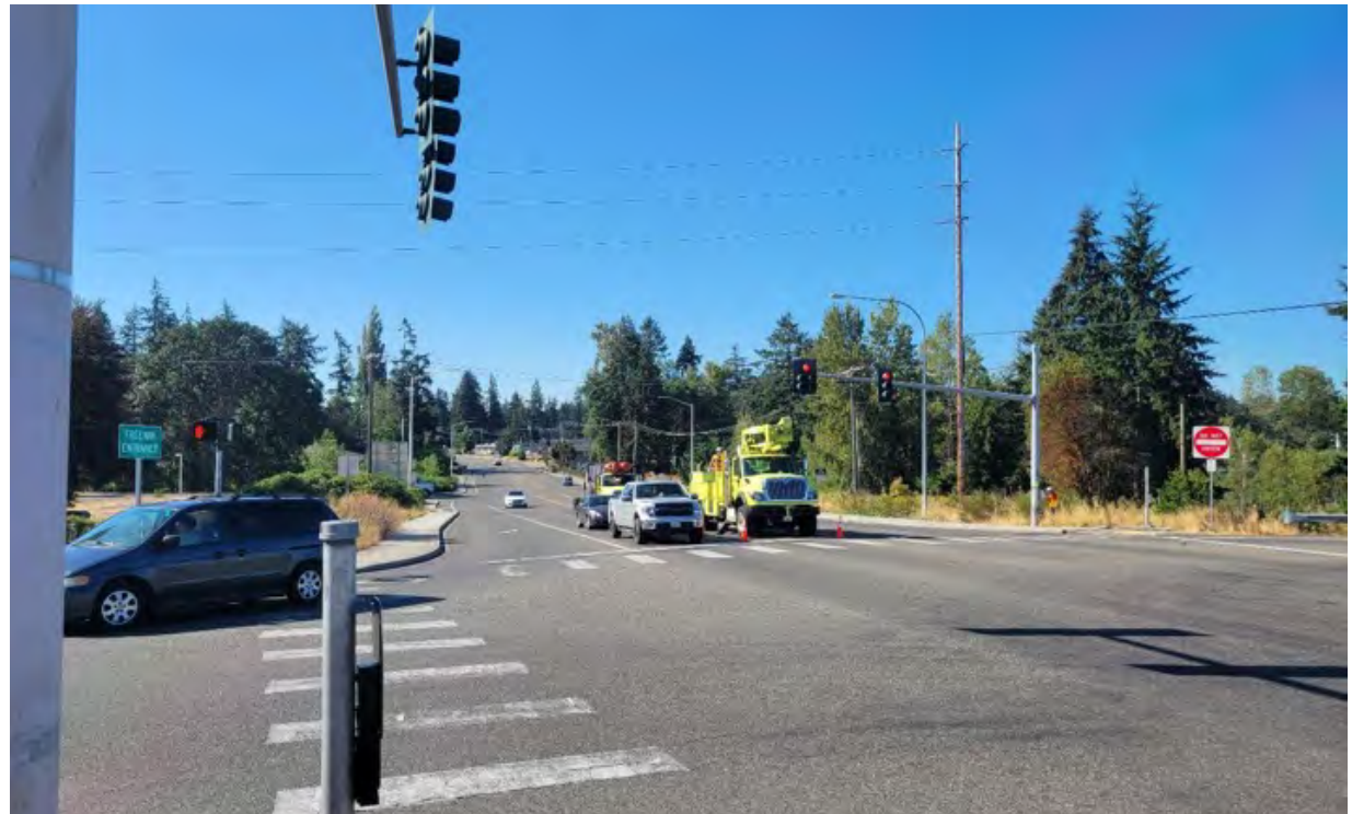
This left turn phase was modified to improve safety and reduce the likelihood of knockdowns of the equipment in the foreground.
