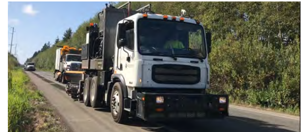
A third party quickly installed the ‘mumble strips’ in a mobile operation using specialized equipment that allows them to configure nearly any type of sinusoidal design
