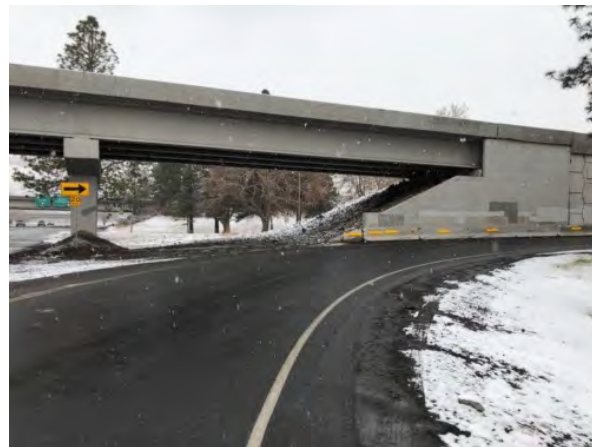
Before: Existing signage and warning devices.
