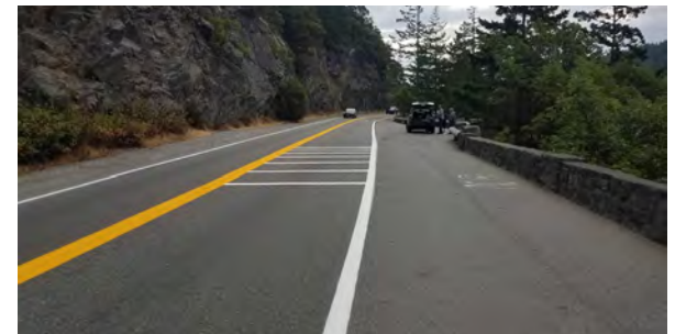
New 20" centerline, 8" edge line, and new transverse rumble strips leading to the bridge.
