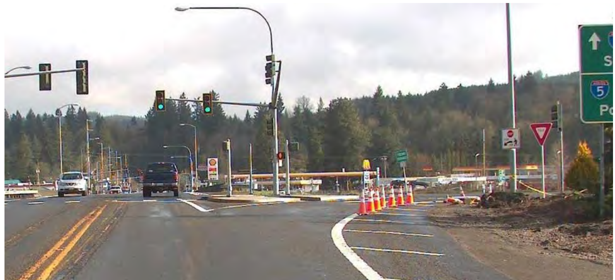
Wavetronix detection installed for SR 411 eastbound traffic approaching the I-5 southbound ramp terminal.
