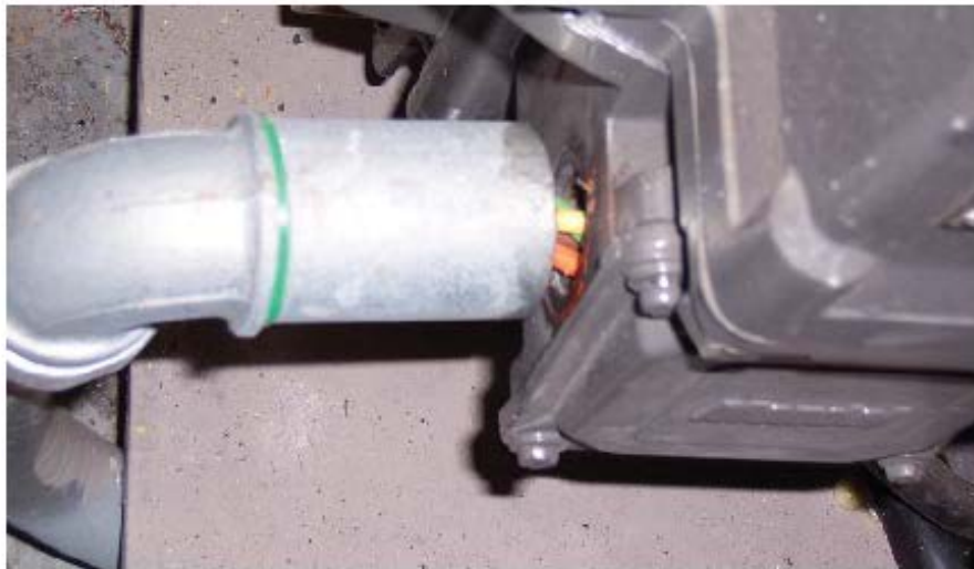
Photo 2 Broken conduit fitting on NE Thruster Brake
