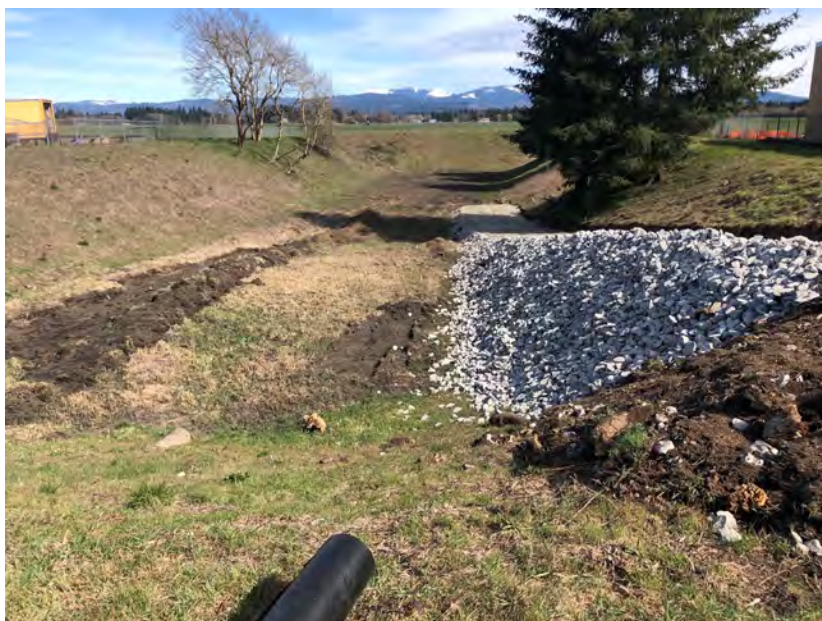
Figure 6. This southwest region pond required over $25,000 in repairs and a new access road. As required in the permit, WSDOT must prioritize repairs to BMPs amounting to more than $25,000 and address them as funding becomes available.
