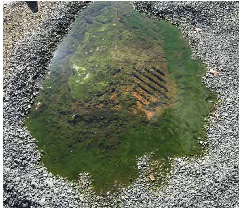
Figure 5. A catch basin overflows due to an illicit connection from a residential area. WSDOT's IDDE program resolves these connections to prevent further negative impacts to WSDOT's stormwater system.
