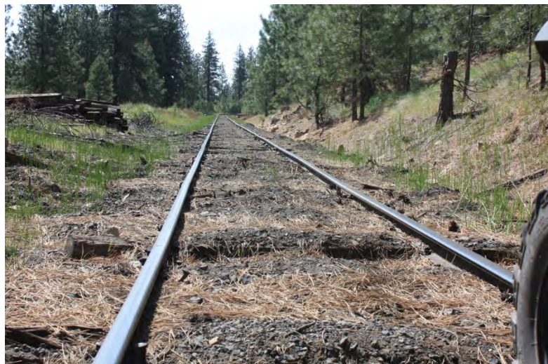
Figure 3.5: Fouled Ballast on CW Branch
