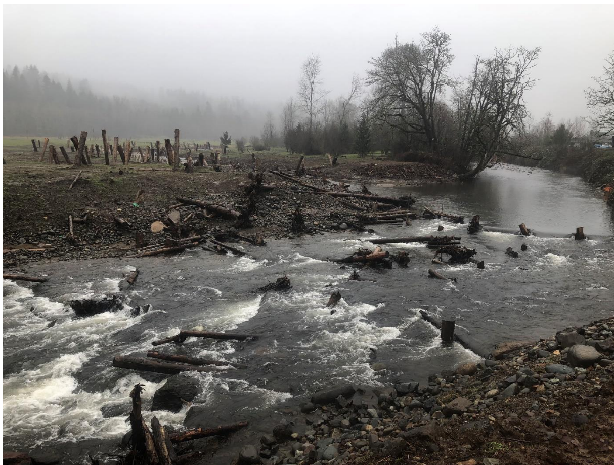
Figure 10-8 Example of Large-Channel Wood Grade Control
