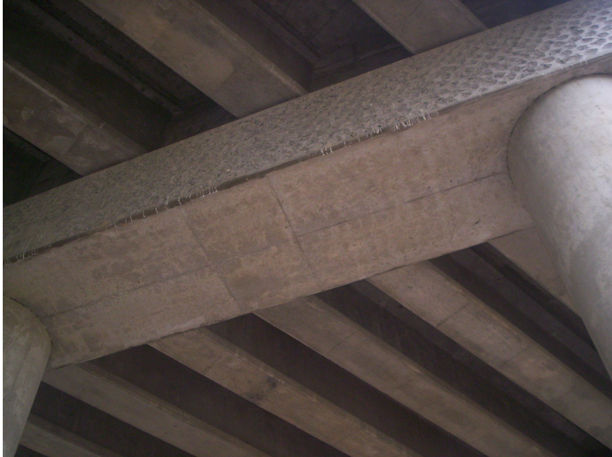
Alternative Spall Pattern Roughening Photo
