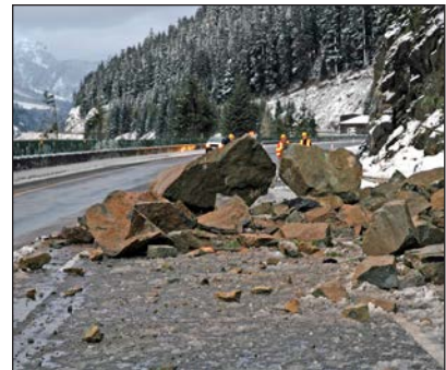
Unstable slopes in the project area regularly lead to rock fall.
