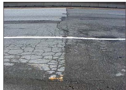
Cracked and deteriorated pavement on I-90.
