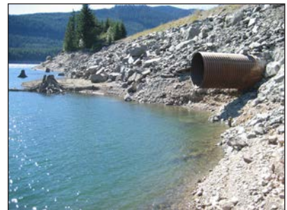
Perched culvert at Resort Creek outlet.
