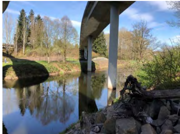
Northbound I-405 to eastbound SR 522 ramp with two piers proposed for removal in the Sammamish River.
