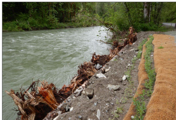
Figure 13. Sauk Side Channel CED, April 2020. This cribwall was installed during an emergency repair in February. Remaining vulnerable streambanks that would be protected are in the background.
