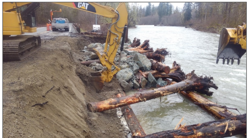
Figure 7. SR 530 Sauk River Side channel CED during construction of the emergency repair in February 2020. This project was constructed during high flows.
