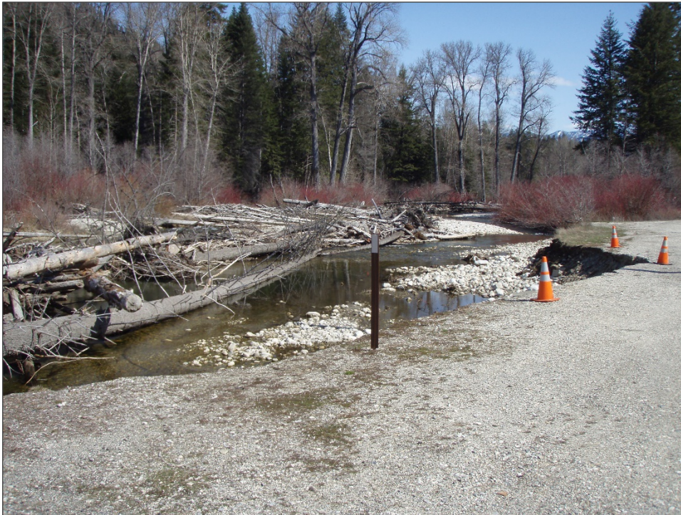
Figure 18. SR 207 Nason Creek embankment failure, April 2011. This CED project is the top priority for the CED program due to high fish benefit, high risk to infrastructure, and a partnership opportunity with the Yakama Nation. The project is planned for construction 21-23 in partnership with the Yakama Nation as the project lead.
