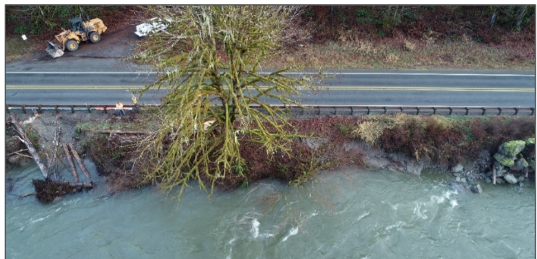
Figure 3. Riverbank failure November 2018.
