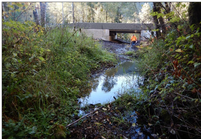
Figure 40. Wooster Creek CED project upstream of the SR 504 crossing, post construction, October 2018.
