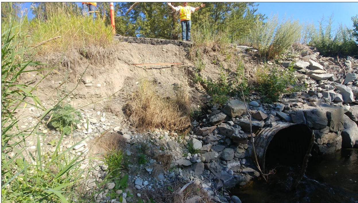
Figure 26. SR 21 Curlew Cr culvert CED, July 2018. Curlew Cr currently approaches the crossing at an angle and erodes the streambank and highway embankment. WSDOT maintenance frequently dredges the inlet of the channel during the frequent emergencies when the culvert gets blocked with sediment.
