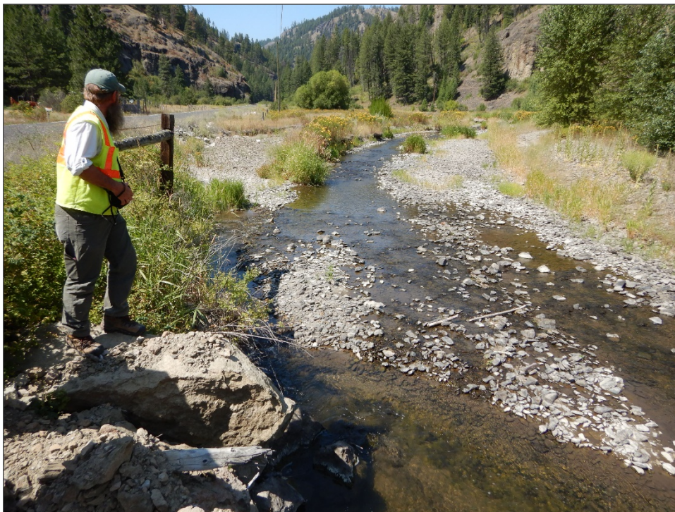
Figure 20. SR 21 Sanpoil River 4 CED, August 2019. The Sanpoil River has been migrating adjacent to the highway at this location and frequently changes course. Eastern Region maintenance staff plan to construct a rock with log toe revetment and bioengineered floodplain bench in summer 2021.
