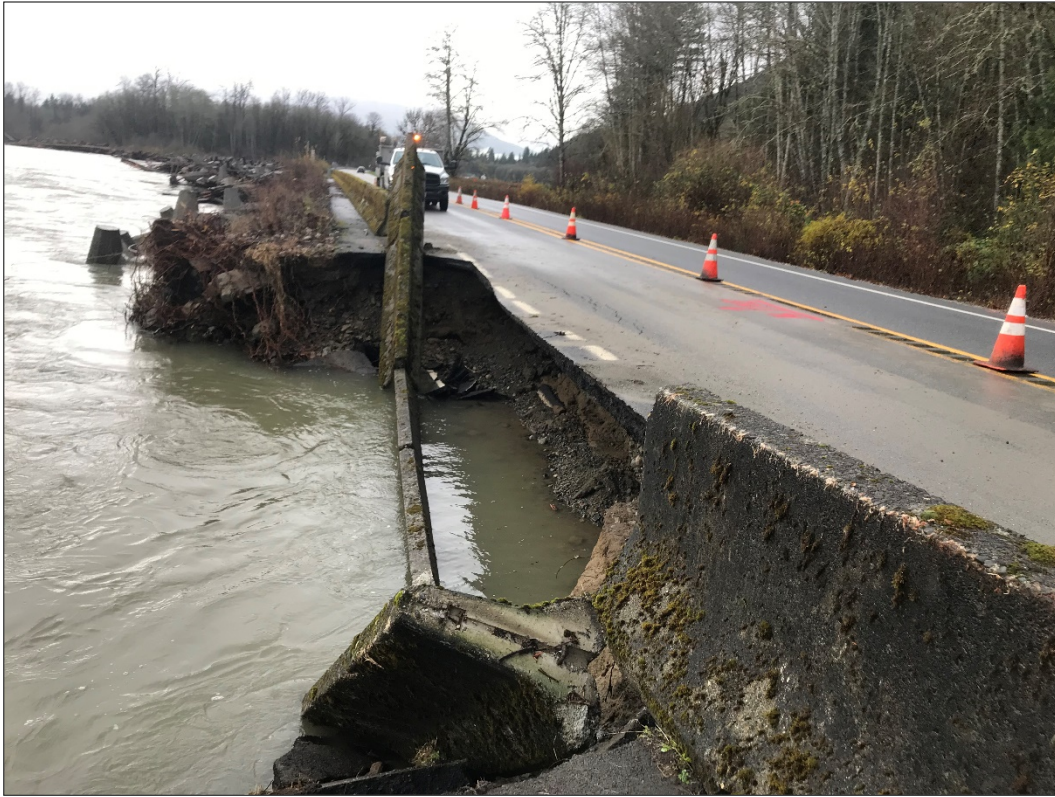
Figure 21. SR 20 Skagit River 2 CED at MP 101 after a high flow event in November 2017. WSDOT is preparing an assessment in conjunction with two other studies to fix this CED.
