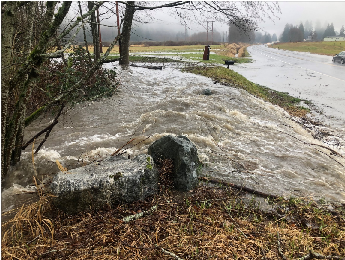
Figure 10. SR 20 Childs Cr CED. Childs Creek overtops a berm and floods SR 20 during a high flow event in February 2021. WSDOT recently completed a site and reach assessment and held a CED concurrence for this CED.
