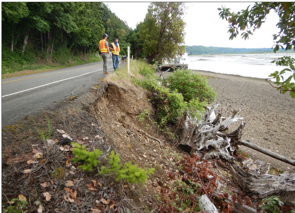
Figure 35. SR 106 Lower Hood Canal Stabilize shoreline CED at MP 5.3, July 2020. This CED consists of a series of small bank washouts along the Hood Canal Shoreline between MP 4.3 and 16.1. This CED is an ongoing effort to address individual sites with various embankment protection techniques including bioengineering and beach nourishment (where feasible).
