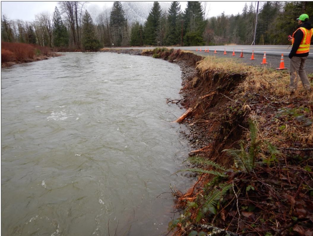
Figure 22. SR 508 Tilton River Morton CED following a high flow event in January 2020, which eroded the embankment upstream of a 2018 CED maintenance repair (shown in background of photo). WSDOT plans to prepare an update to the recently completed 2019 site and reach assessment in order to address current conditions.
