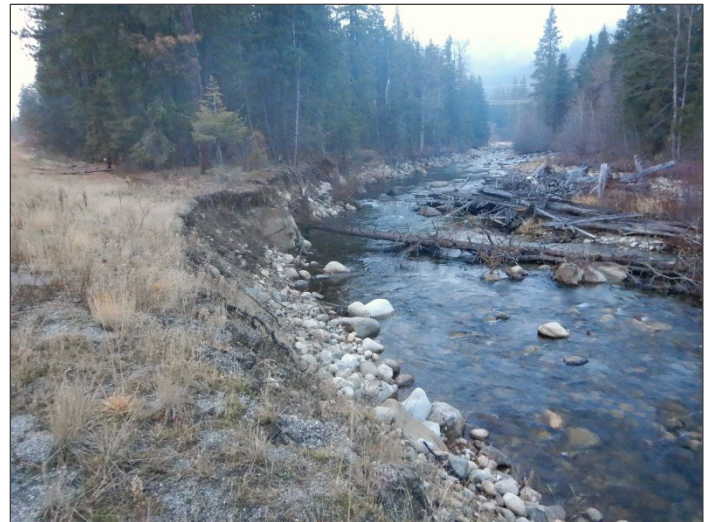
Figure 28. US 2 Nason Cr Kahler CED, November 2019. This site is actively eroding toward US 2.
