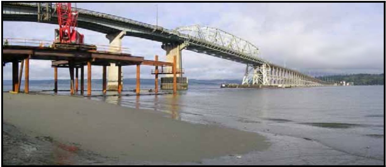
Figure 2. Photograph of Hood Canal Bridge Study Site Showing Temporary Work Trestle Below Eastern Approach of Main Bridge Span at Low Tide
