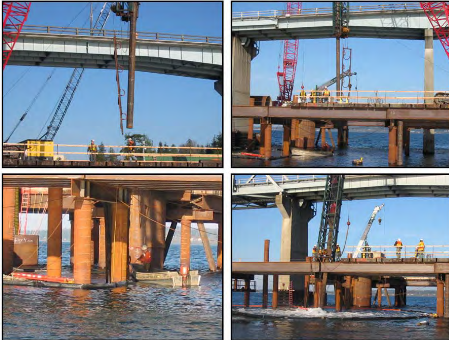
Figure F 8. Type IU unconfined Bubble Curtain and Batter Pile, Pile and Bubble Curtain Lowered into Place, Air Connection to Bubble Rings, and Batter Pile Driving with Bubble Curtain in Place (hydrophone float visible at lower right)
