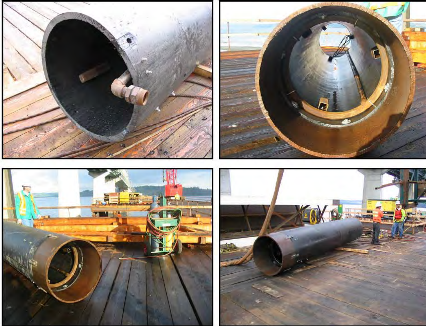
Figure F.4. Type II Confined Bubble Curtain Sleeve Showing Air Supply Connection, Bubble Ring, Metal Extension to Contact Substrate
