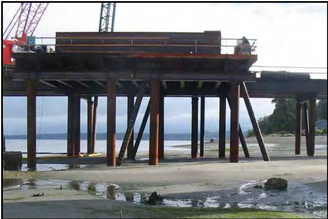
Figure 3. Plumb (vertical, 24-in. diameter) and Batter (angled, 16-in. diameter) Piles Supporting Temporary Work Trestle at the Eastern Approach of the Hood Canal Bridge
