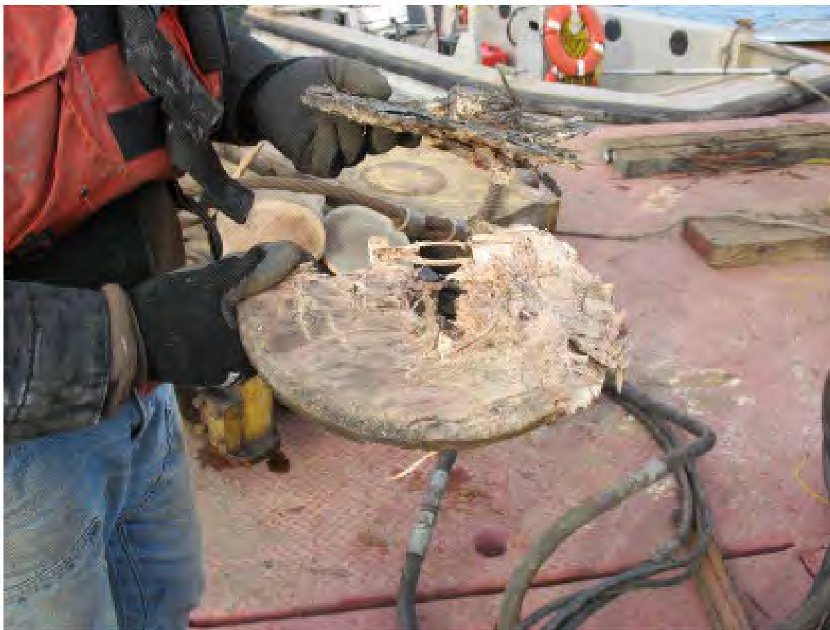
Figure 7: Fractured and compressed wood pile cap after being used on piles 5, 6, and 7 (photo courtesy of Washington State Parks and Recreation, R. Johnson)
