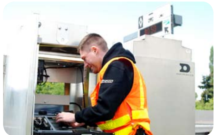
WSDOT HOT lanes technician Allen Mushatt checks the electronic equipment cabinet, saying, "For the most part, the system monitors itself."
