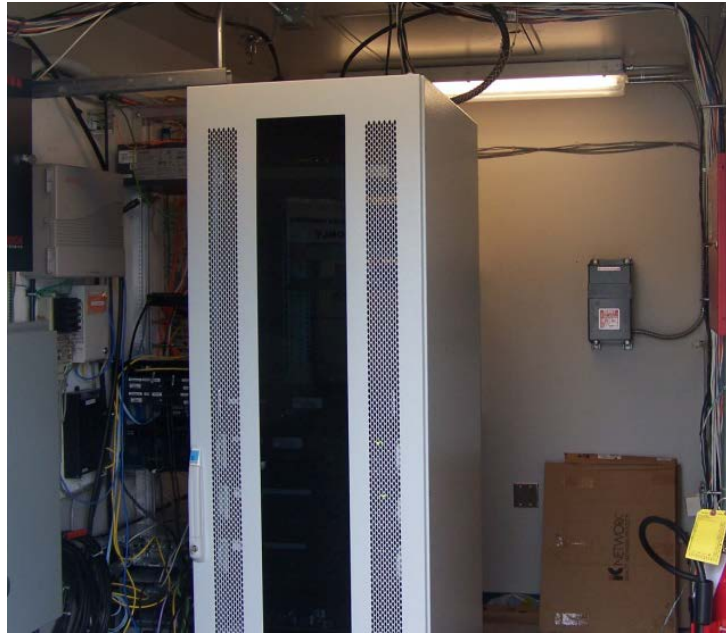
Clinton Ferry Terminal IT Equipment Network Room Exhibit 400-10
