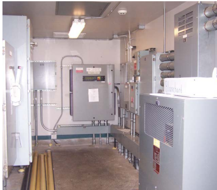
Clinton Ferry Terminal Electrical Room Exhibit 400-11
