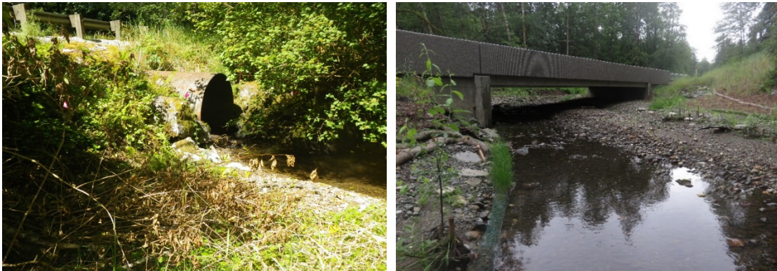
Exhibit 1: SR 9 Lake Creek. Prior to restoration, the culvert was undersized and water was restricted. Post-construction, stream is free to move through the culvert and buffers are restored with native plants.
