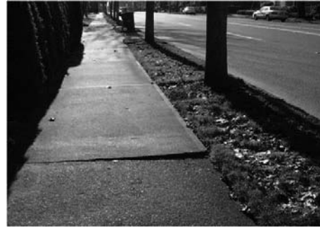
Unacceptable Pedestrian Access Route
