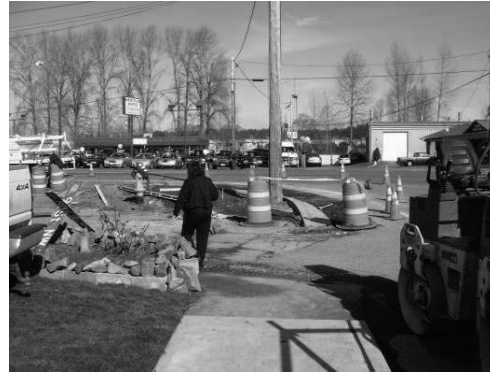
Does Not Meet ADA Requirements
