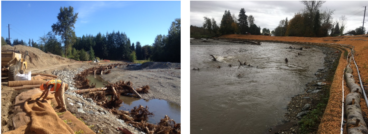
Exhibit 13: SR 92 Pilchuck River Chronic Environmental Deficiency Repair – constructing bank protection and bank protection during first storm.
