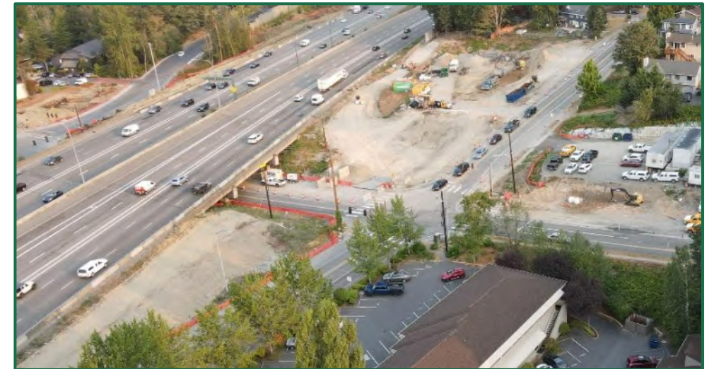
Construction is underway on a northbound onramp to I-405 at the intersection of 132nd Street and Totem Lake Boulevard
