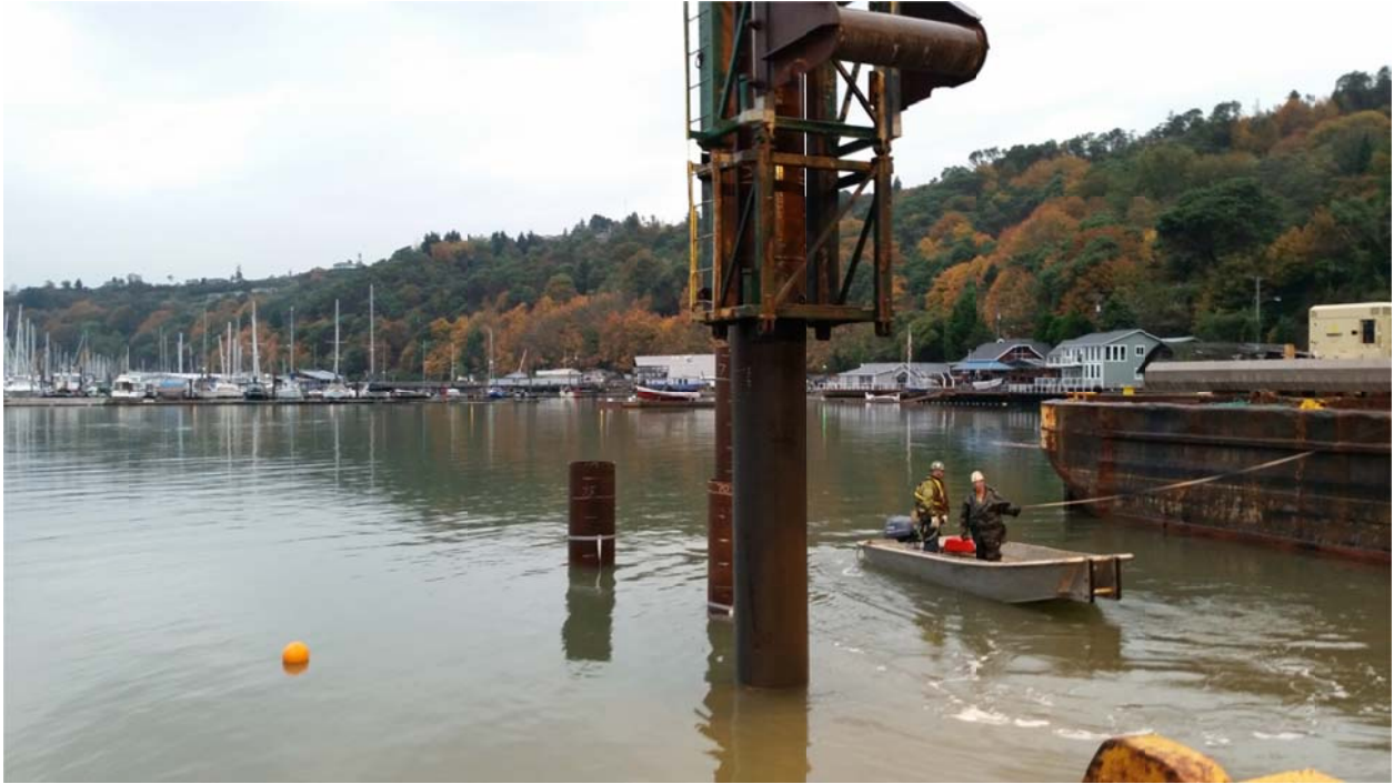
Figure 3a. Photograph made on October 30 th of the 3 piles shown in order of nearest to farthest: Mandrel Pile, Double Pile and Control Pile. Buoy marker on left shows approximate position of the VLA.
