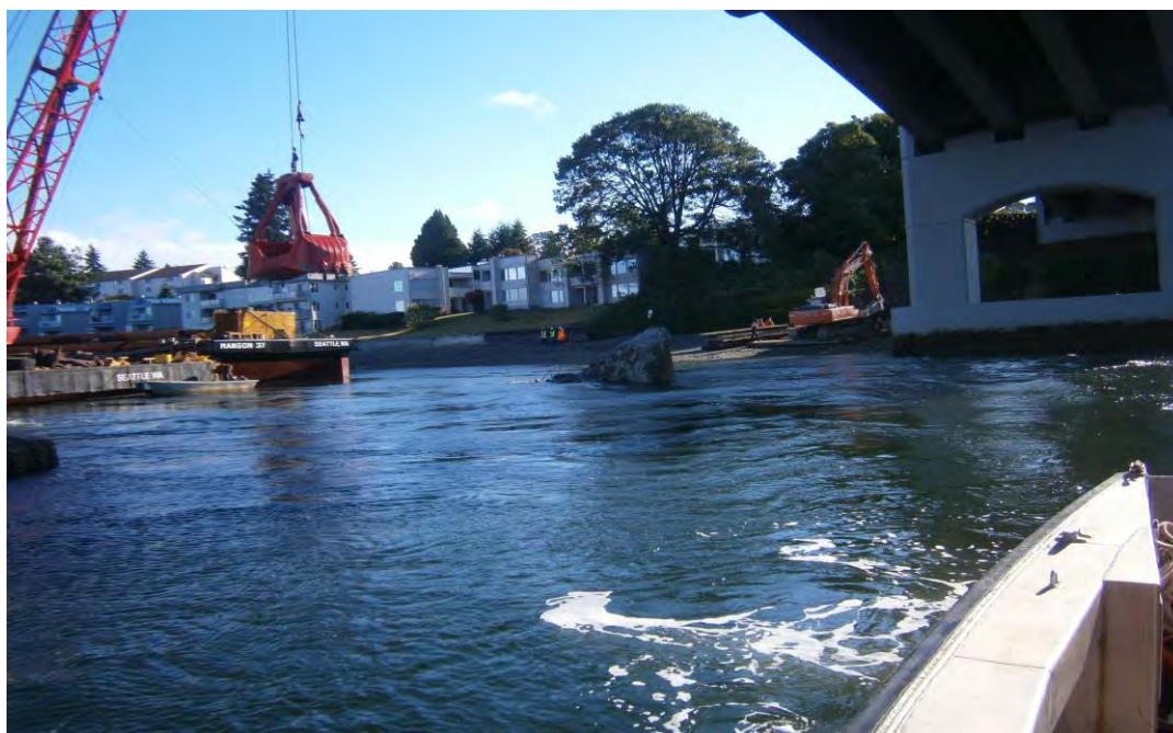
Figure 7: Machinery to be used for debris removal of debris after Ram Pier 5A Demolition
