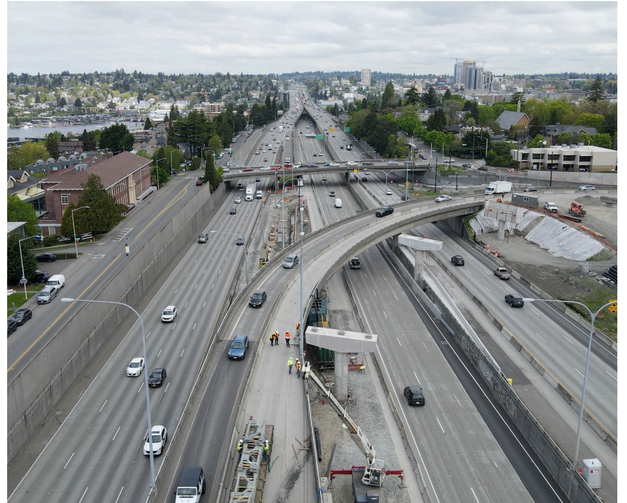
The concrete crossbeams shown will be where the new steel bridge girders are placed.
