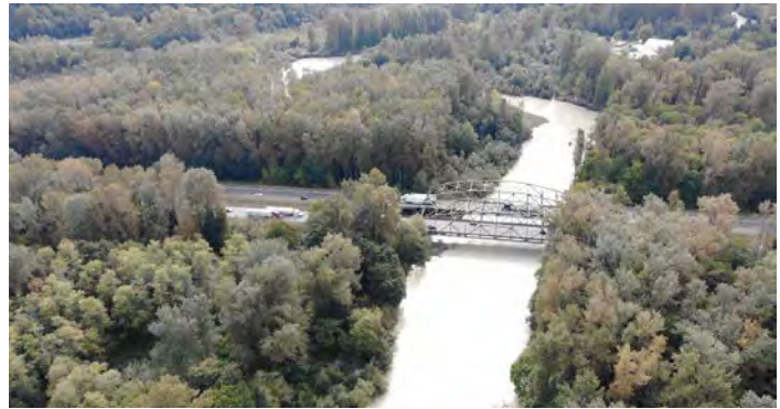
WSDOT considers both I-5 bridges over the Nisqually River bridges to be in fair condition with more than 30 years of remaining service life.
