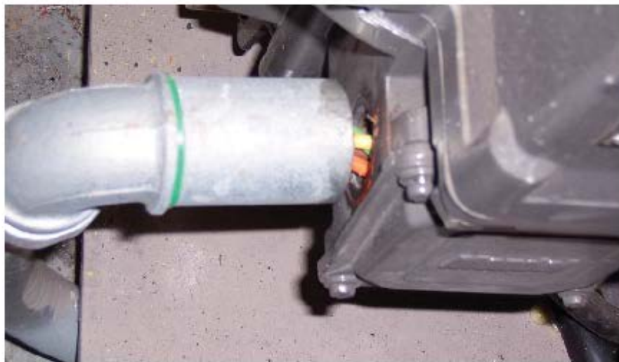
Photo 2 Broken conduit fitting on NE Thrustor Brake
