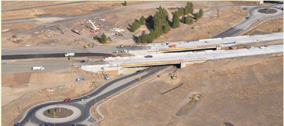
A bird's-eye view of construction at Freya Street as part of the US 395/North Spokane Corridor project. This portion of the larger NSC project was operationally complete in October 2018.
