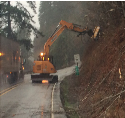
Top: WSDOT crews take a closer look at the detachable truck bed which saves time and work associated with unloading and loading trucks during guardrail repair projects. Middle: The guardrail rake innovation allows one equipment operator to clean debris from under guardrails—a task that used to require three manual laborers. Bottom: The hydraulic brush mower attachment allows one equipment operator to clear brush and tree limbs efficiently.
